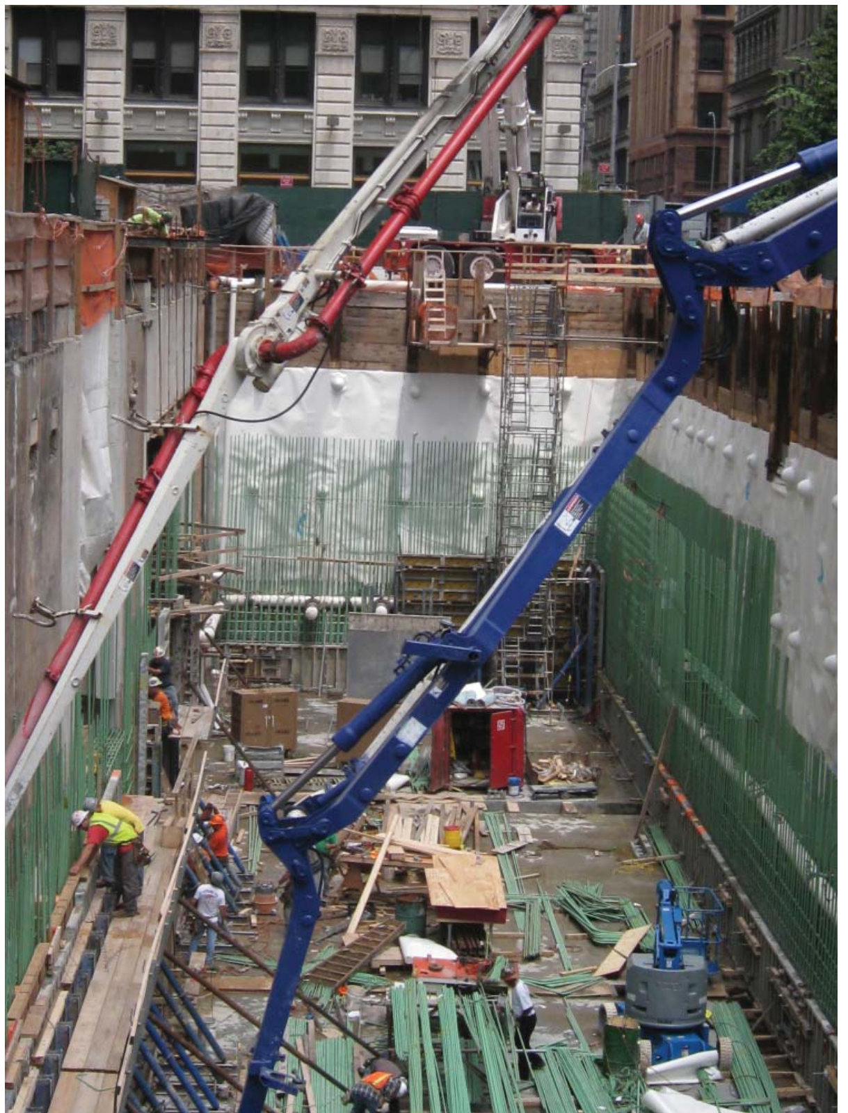
Workers building the cogeneration plant's foundation. The excavation walls stretched down to a depth of 50 feet below ground, giving some sense of the plant's enormity.
